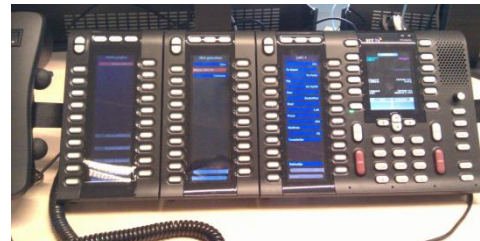
Figure 3.3.7: A phone in a control room
