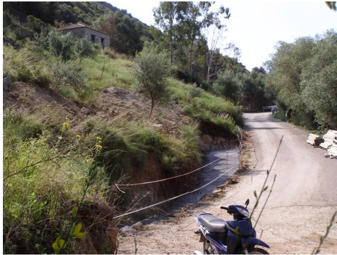
Figure 6: The bulldozer cut adjacent to the road, view from the northwest (photo: author)
