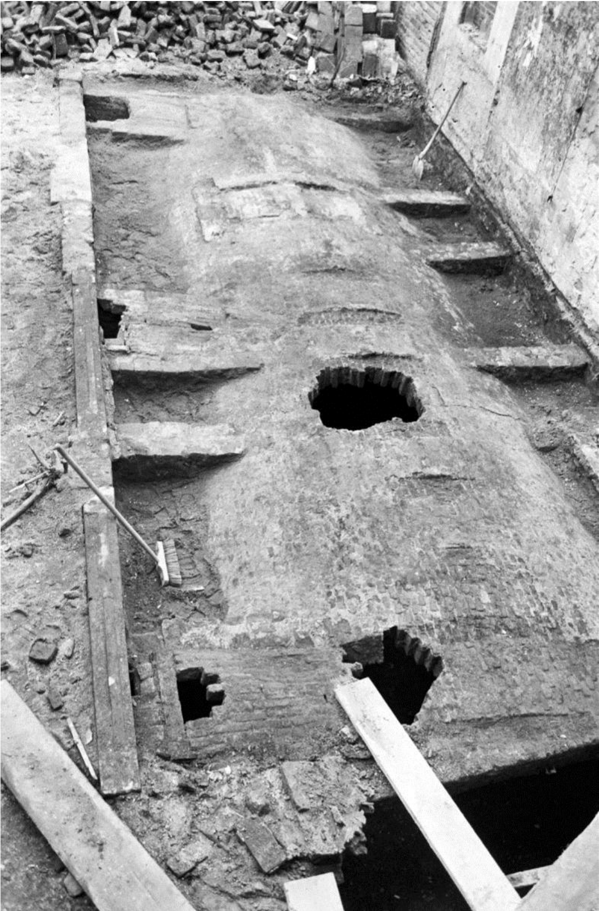
Figure 5.12 A rare top view of a vaulted cellar belonging to Noordenbergstraat 9 (1621) in Deventer. The photo clearly shows how the cellar forms a closed brick space in the ground. The hole in the vault will be of recent date, possibly to realize an internal passage. (source: www.rijksmonumenten.nl ; photographed by: Berends, G., April 1971 | License: CC-BY-SA-3.0-NL (wiki)).
