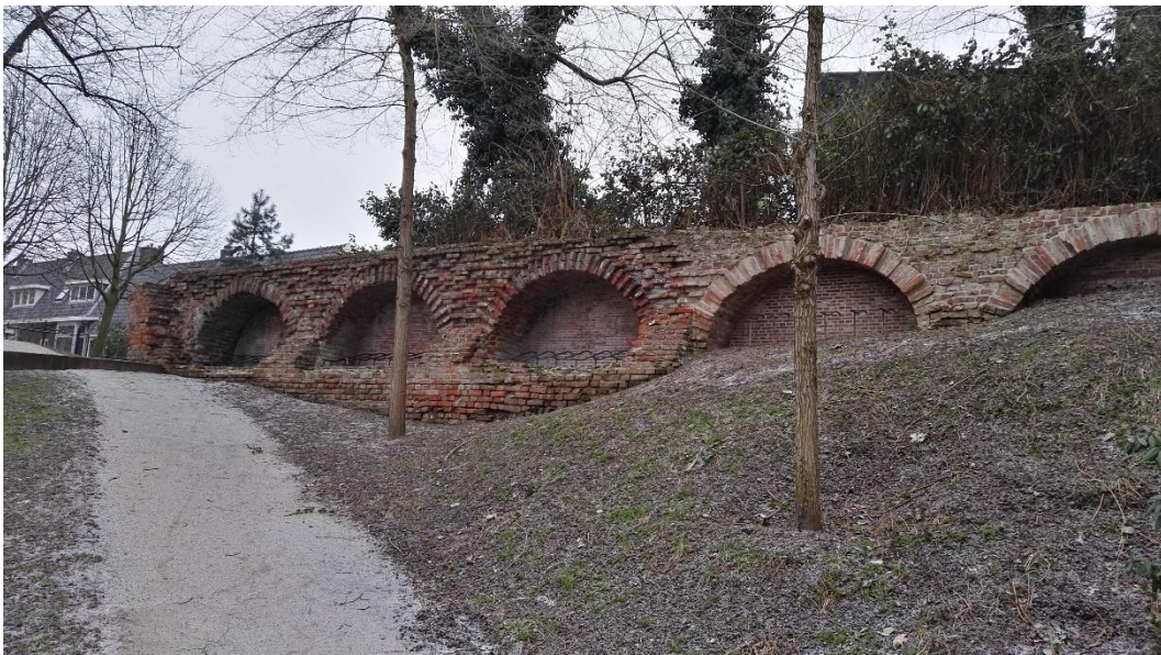
Figure 9, still standing stretch of medieval town wall on the Nobeldwarsstraat. Here we see the arch construction on the town side. The shield wall has been stripped off in the 19 th century and a supportive wall has been constructed on the town side closing off the arches.
