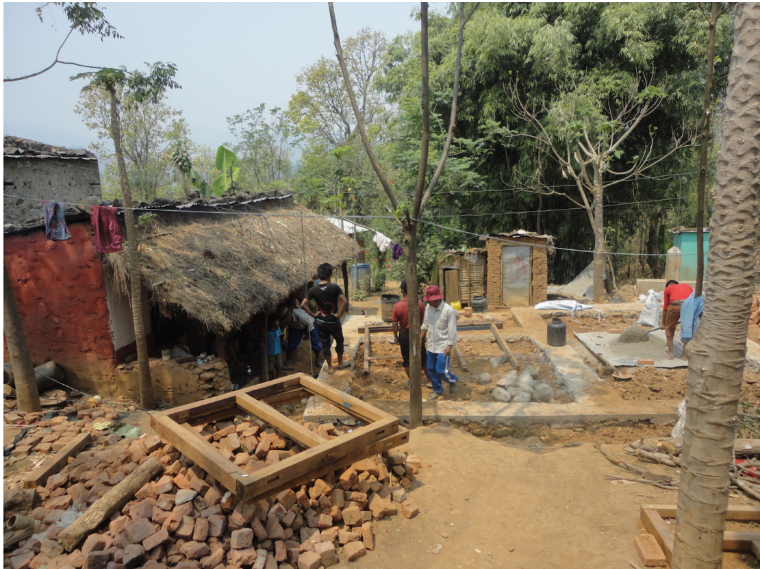
Fig. 2.3. Ek Bahadur's new government funded house under construction beside his old house (left), one of only two Gandharba houses that were granted this year (2014) in comparison to seven from the previous year. Ongoing speculations are that in 2015, every Gandharba family still awaiting their grant will be fulfilled.
