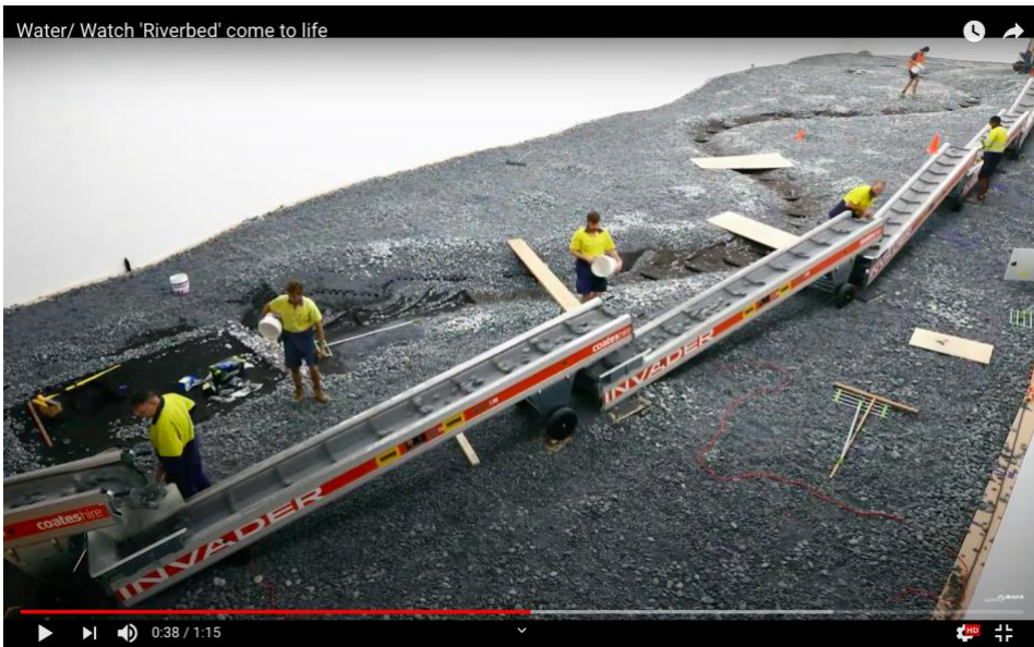
Fig.27: Three screenshots of the YouTube video “Water/Watch ‘Riverbed’ come to life”, which is a 1m 15sec time lapse video of the construction of Riverbed , 2019-2020, at the Gallery of Modern Art, Brisbane, Australia.
