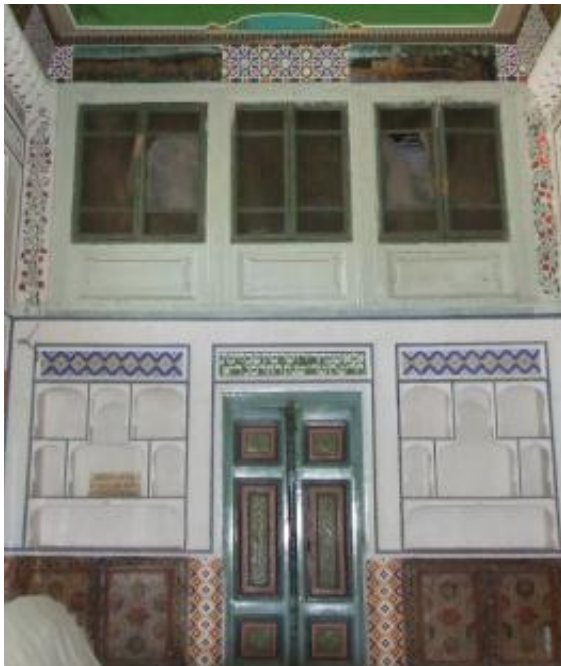
Figure 56: Women's section, above main door, Rafael Abramov house, Samarkand. (The Center for Jewish Art).
