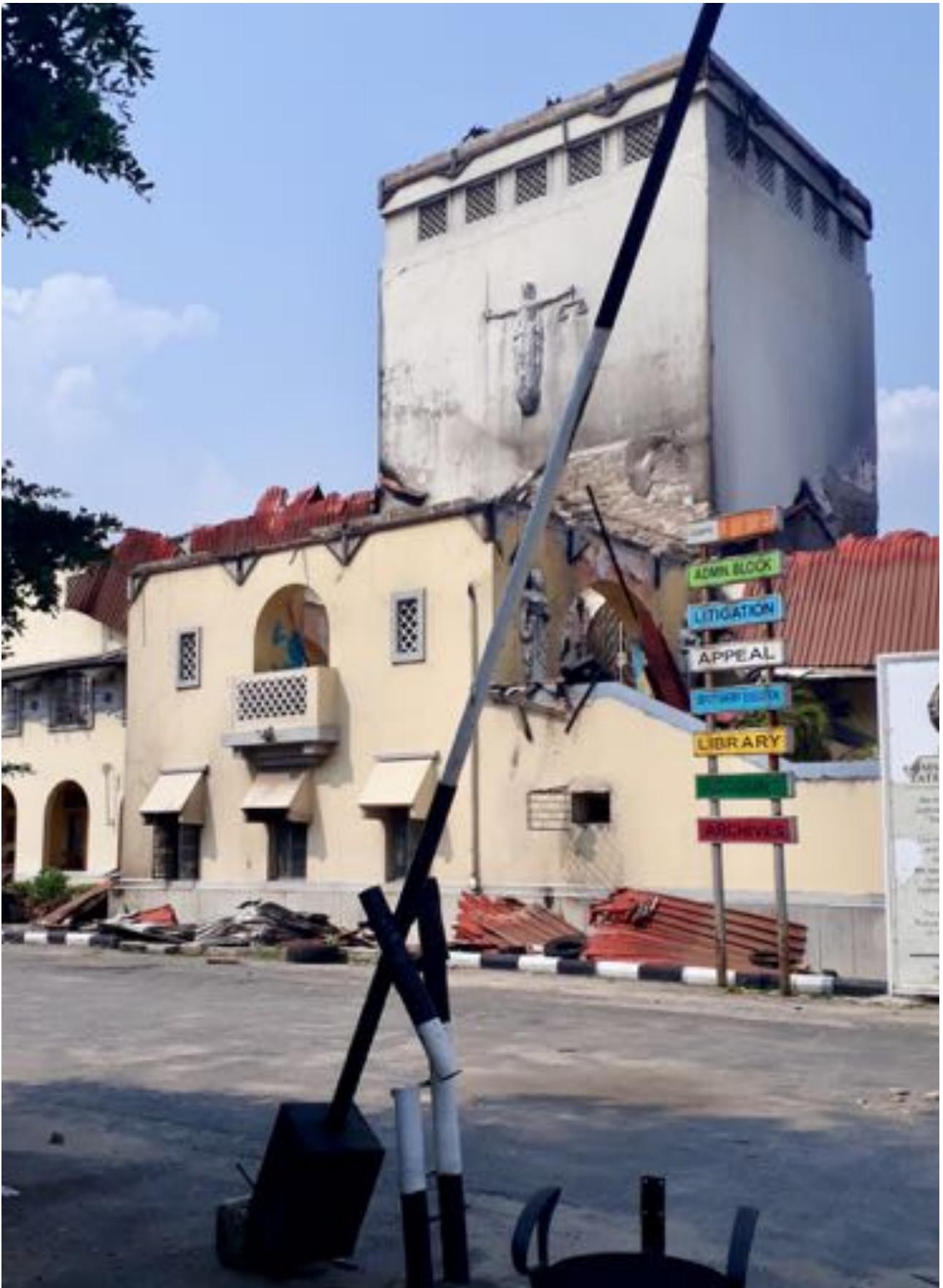
The partly burnt Federal High Court building in January 2021. (Photograph: Femke van Zeijl)
