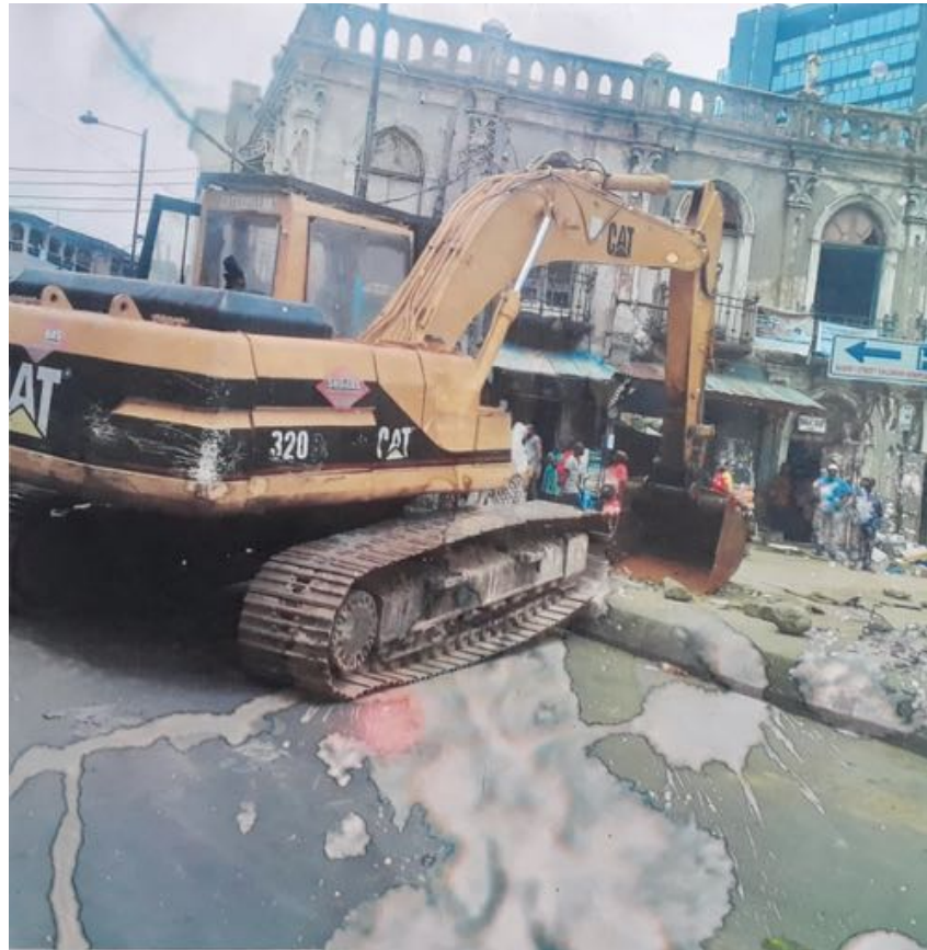
An earlier attempt to demolish Ilojo Bar in 2016 which was averted. (Source: a resident)
