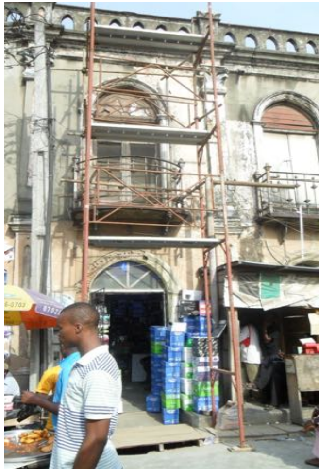
Scaffolding put up at Ilojo Bar early 2012 for the survey. (source: Legacy)
