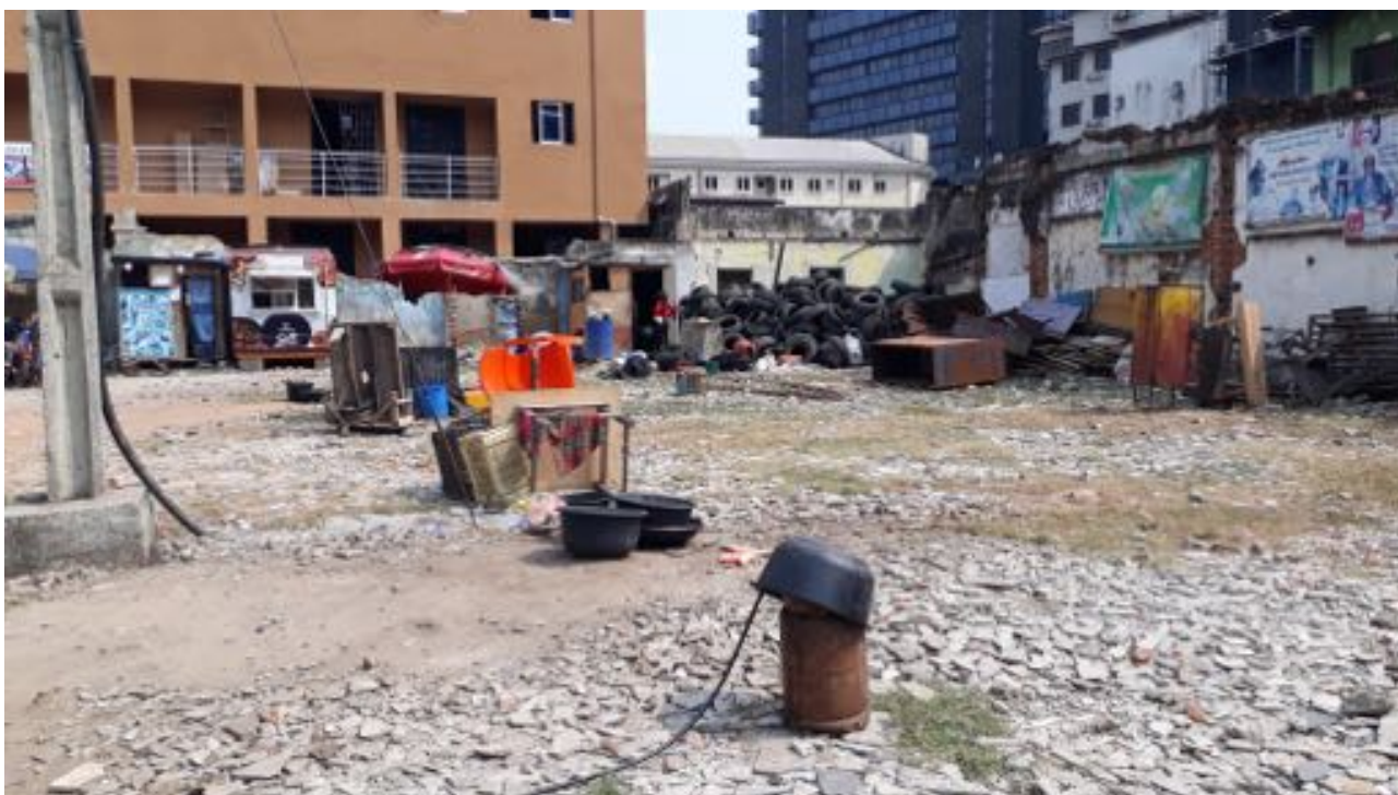
The state of the demolition site of Casa do Fernandez in February 2021. (Photographer: Femke van Zeijl)
