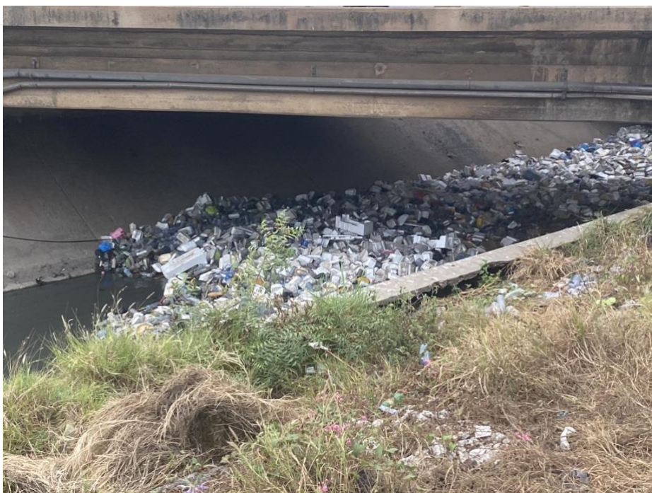
These pictures depict the current situation in Accra regarding SUP waste that blocks drainage systems, causing flooding. Most of the waste in the gutters is plastic.
