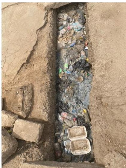
Figure 1: blocked gutters in Accra
