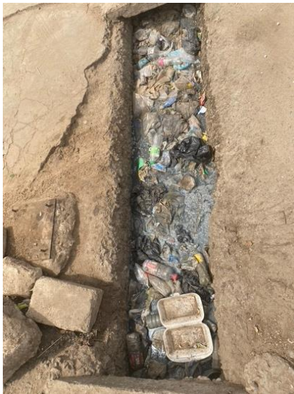
Figure 1: blocked gutters in Accra
