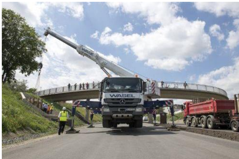
Figure 15. The installation of 5 pieces of the Roman aqueduct along the new road (Claßen and Vollmer-Köning 2021, 4).
