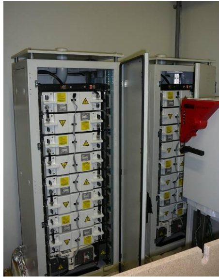
Figure 2: Example of a storage system (Li-ion, from SAFT)
