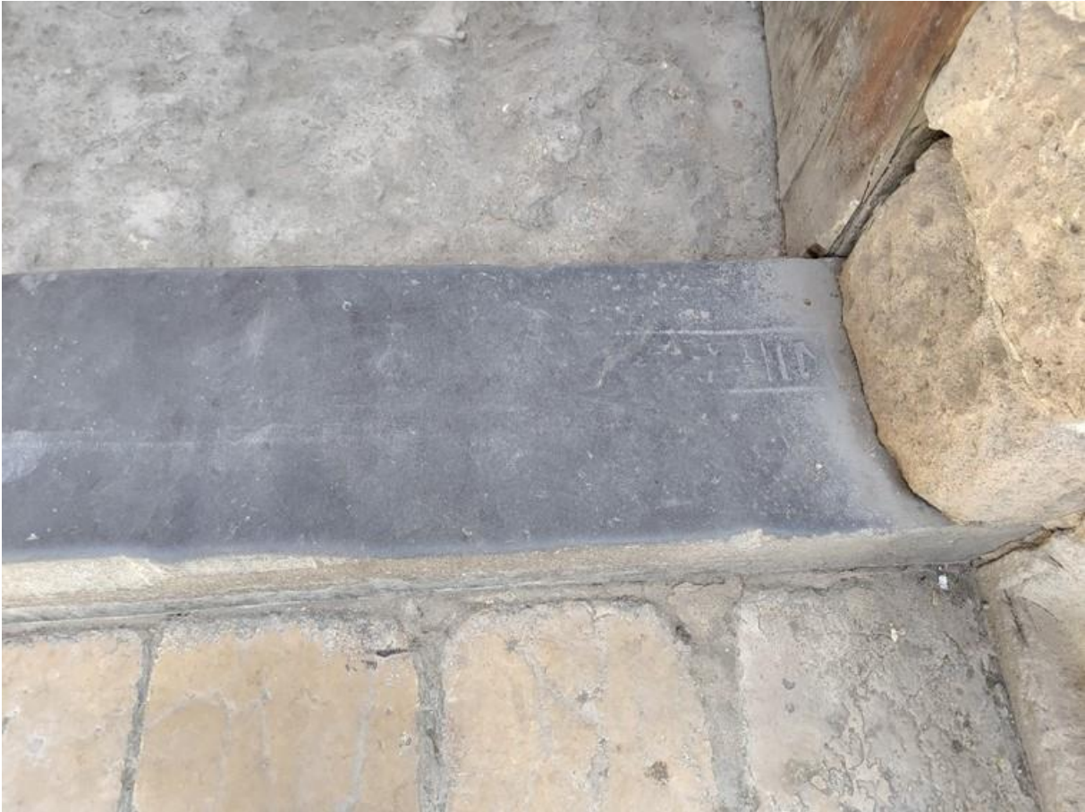
Figure 5. The right block of the threshold showing hieroglyphs at the main entrance of the Aqsunqur Mosque (1346 AD). The photo is taken from the road (PHOTO BY THE AUTHOR).
