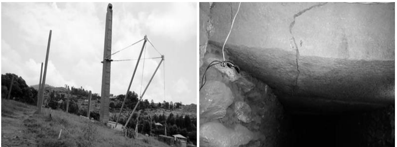
Fig. 72: Cracks in the slabs supporting the doorway to Mausoleum (Hagos, 2018; 301) Destabilized Stele 3 and current support system in place (Hagos, 2018; 302)
