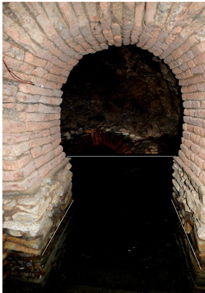
Fig. 73: Picture of water flooding the Tomb of the Brick Arches, reportedly standing over a meter high (Walker 2019).
