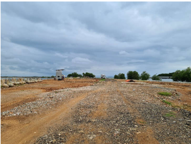
Figure 48. New reclamation project in Pantai Mutiara for the construction of a luxury hotel.
