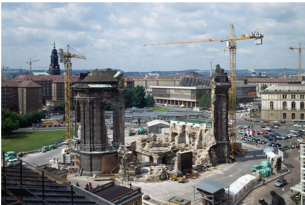
Figure 4.1. The Frauenkirche at the start of the rebuilding process, after the debris removal. Source: Stiftung Frauenkirche Dresden.
