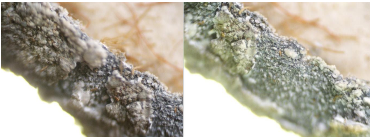
Figure 16. A microscopic view of the pin shows the corrosion and tiny sand particles on the metal frame.
