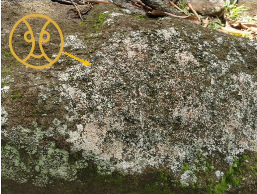
Figure 3.3.1.3. Efflorescence on rock with petroglyph. Due to the chemical process, the petroglyph on this rock in Le Parc Archéologique des Roches Gravées is no longer recognizable. Therefore, the original drawing is shown in orange in the upper left (Photograph and drawing: A. Dekker).
