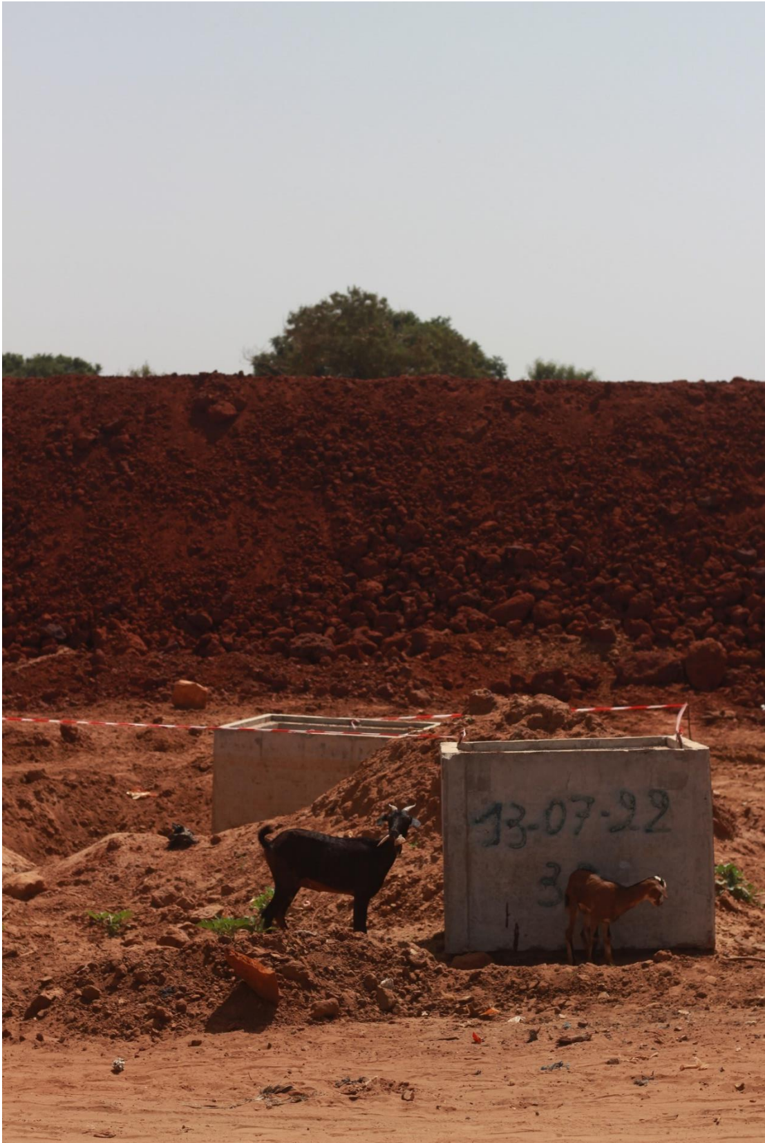
Photograph 10 - The new plant-animal-soil relations. The trainline's bank of quarried soil clears through the town and fields.
