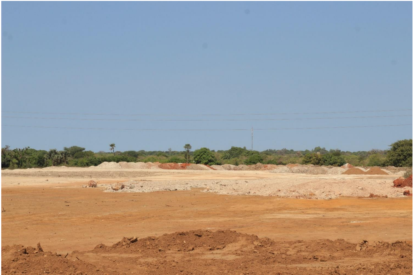
Photograph 8 – After: The foundations for a new TER Station laid out over the previously imaged farmer’s tomato field.
